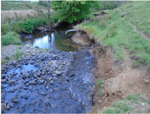
Figure 3.19 : Knickpoint and bank erosion (facing downstream)
