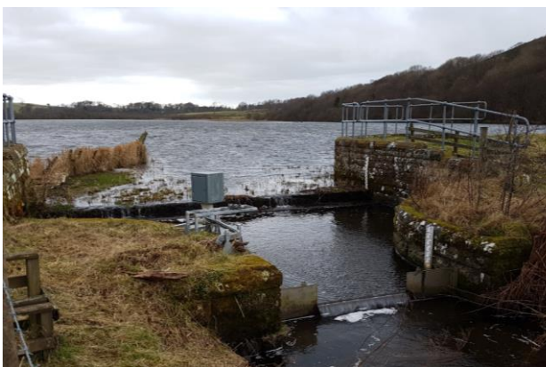
Figure 4-1: Over Water overflow
