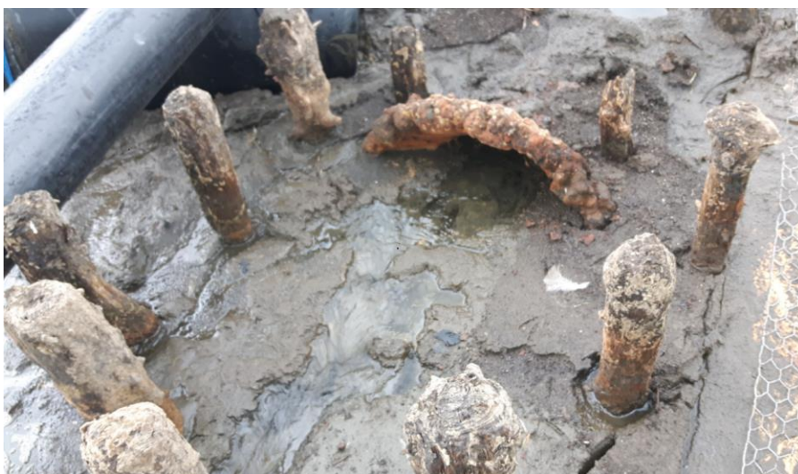
Figure B-7: The partially blocked state of the Over Water intake pipe that transfers water to Chapelhouse, observed during the 2018 drought
