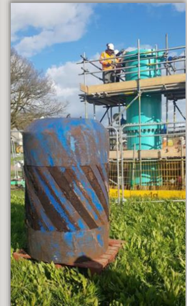
A used 'pig' covered in the iron and manganese picked up from the pipe
