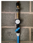
Meter housing assembly incorporating all the required fittings
