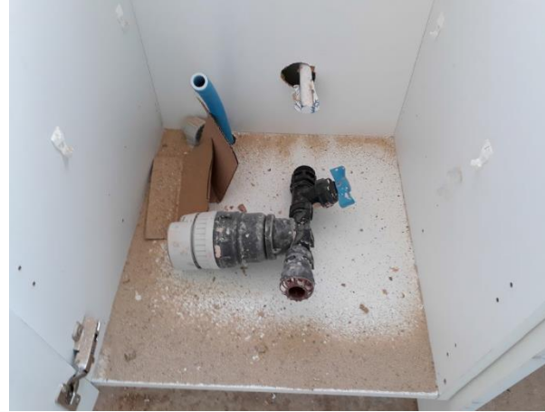
Internal meter install poor practice
