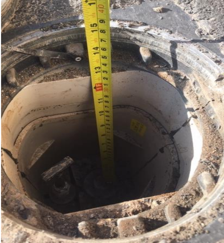
Non compliant boundary box
