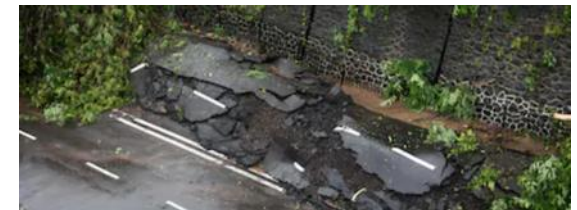
Landslips etc. causing health and safety risks, and supply interruption
